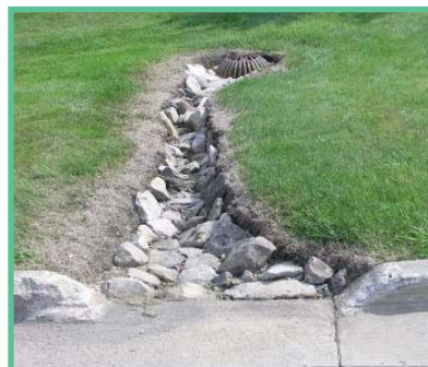
Unstable flow path.
